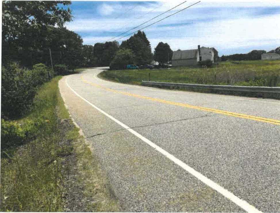
Photo 1 (06-20-18): Facing south Sawyer Road crossing of the culvert. Crack on surface of the road may be due to the presence of culvert.
