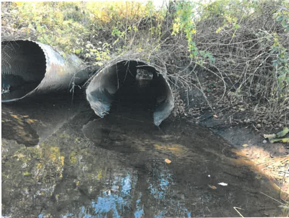
Photos 3 (10-22-18): Looking down the barrel of the westerly inlet of the two Inlet culverts. Culverts' inlet invert has rusted away and the pipes are in poor condition.
