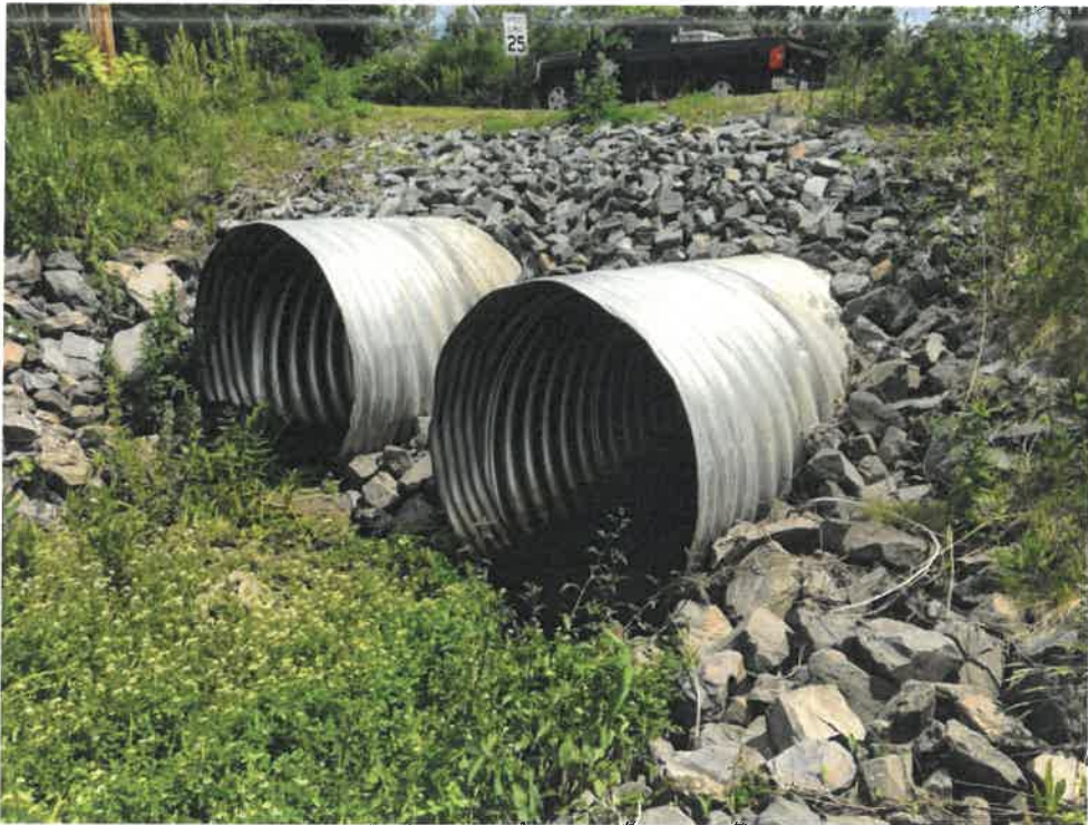
Photo 2 (06-20-18): Inlet of two, 54-inch corrugated aluminum pipes located northerly of Willow Brook. Westerly (right) pipe is set lower to carry the primary flow. Inlet has a well armored rip rap apron and headwall.
