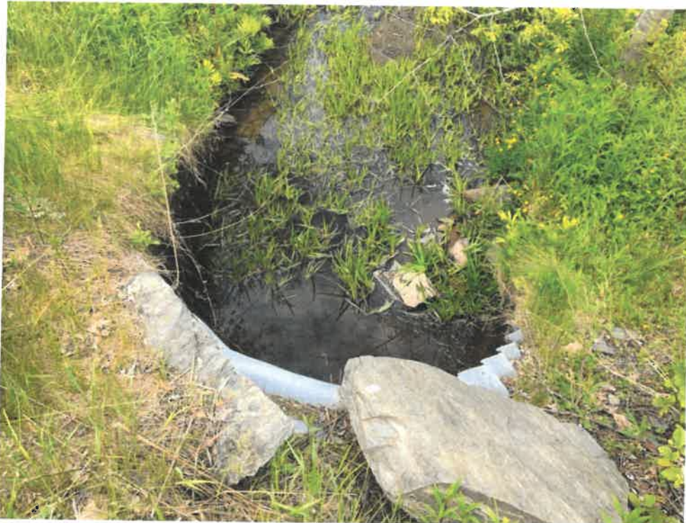
Photo 8 (06-06-18): Overhead view of culvert outlet with stones and vegetation in the outlet channel.
