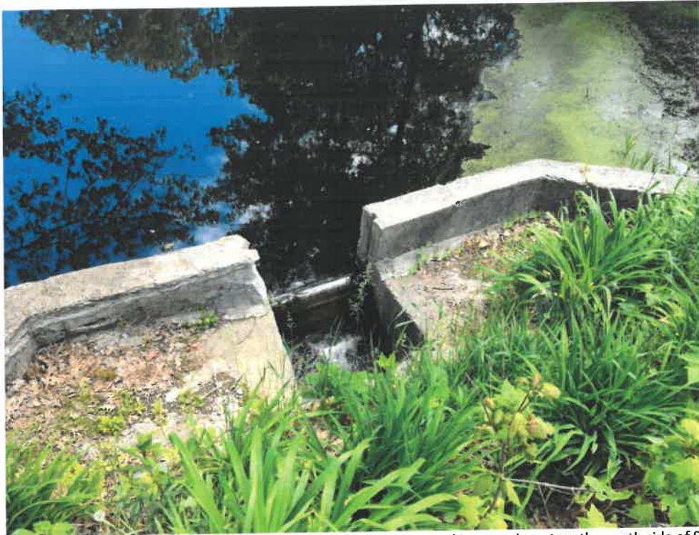
Photo 3 (06-06-18): Concrete wall with wooden board weir outlet to pond impoundment on the south side of Spurwink Avenue.
