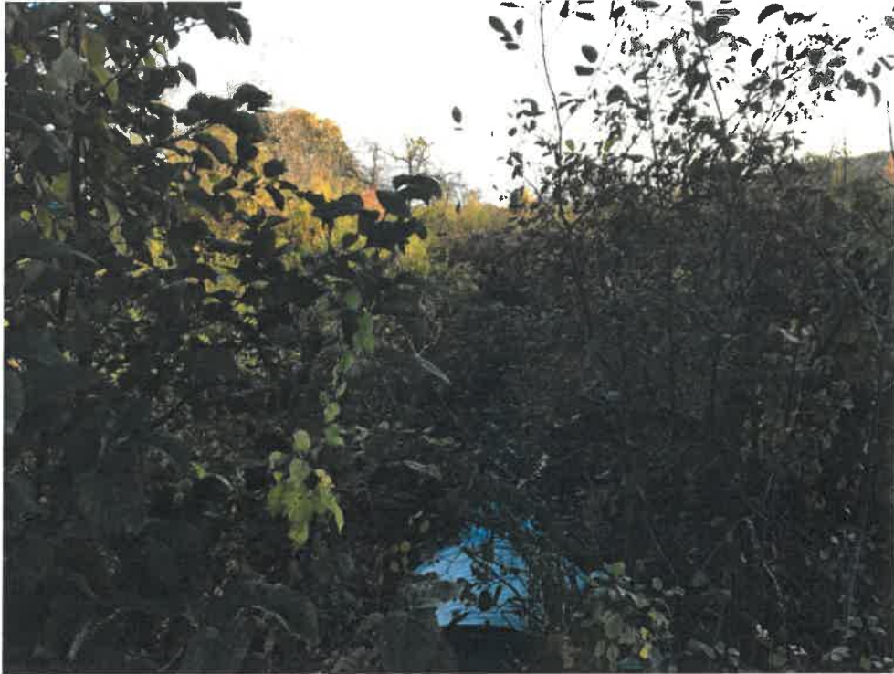
Photo 7 (06-06-18): Looking northeast at the flow from the culvert outlet on east side of Spurwink Avenue. Downstream vegetation obscured channel at the time of the photo.
