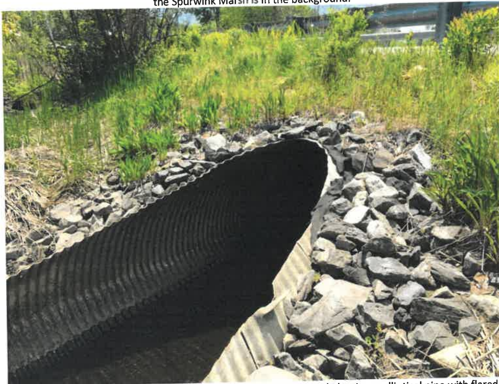
Photo 2 (06-06-18): Submerged inlet of 6-foot wide by 5-foot high corrugated aluminum elliptical pipe with flared end and rip rap headwall. Additional headwall rip rap should be added to the headwall.
