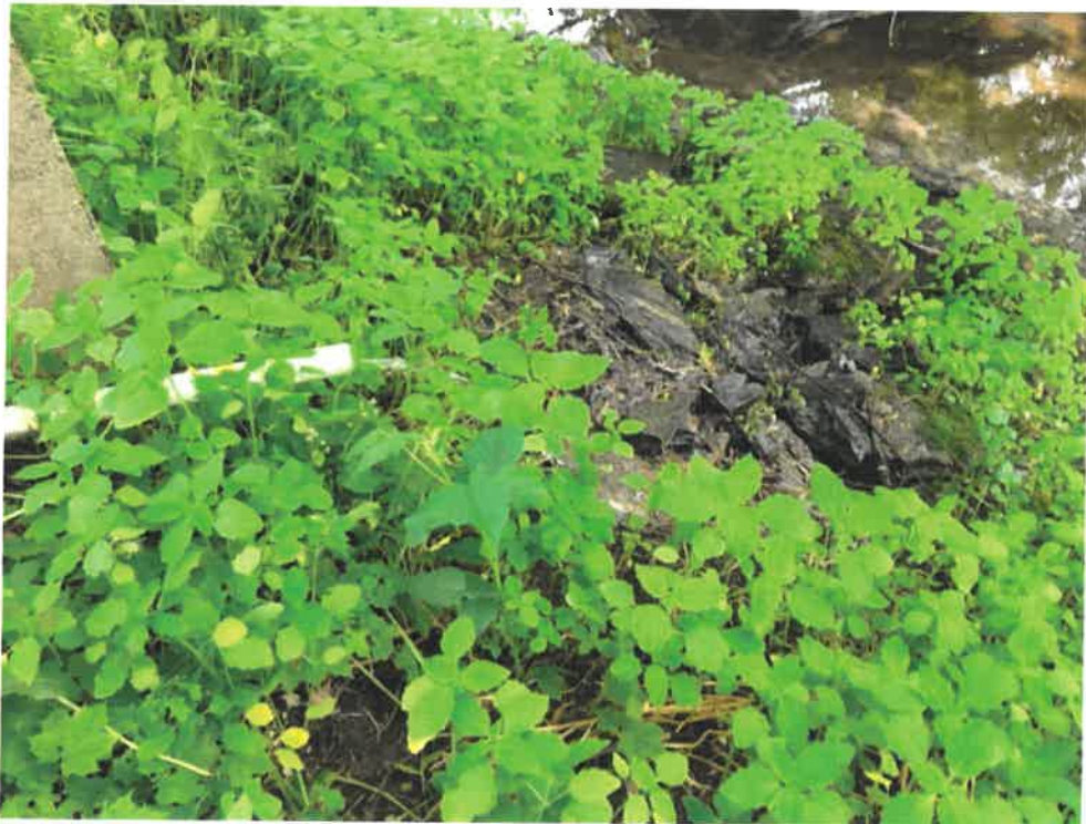
Photo 5 (06-06-18): Facing west at the east end of the concrete wingwall on the south side of the culvert inlet. Small diameter white pvc pipe is conveying groundwater flow directly into Trout Brook despite being a relatively dry weather period. Trout Brook receives surface flow and groundwater flow from residential neighborhoods and other developed areas in close proximity to the stream.
