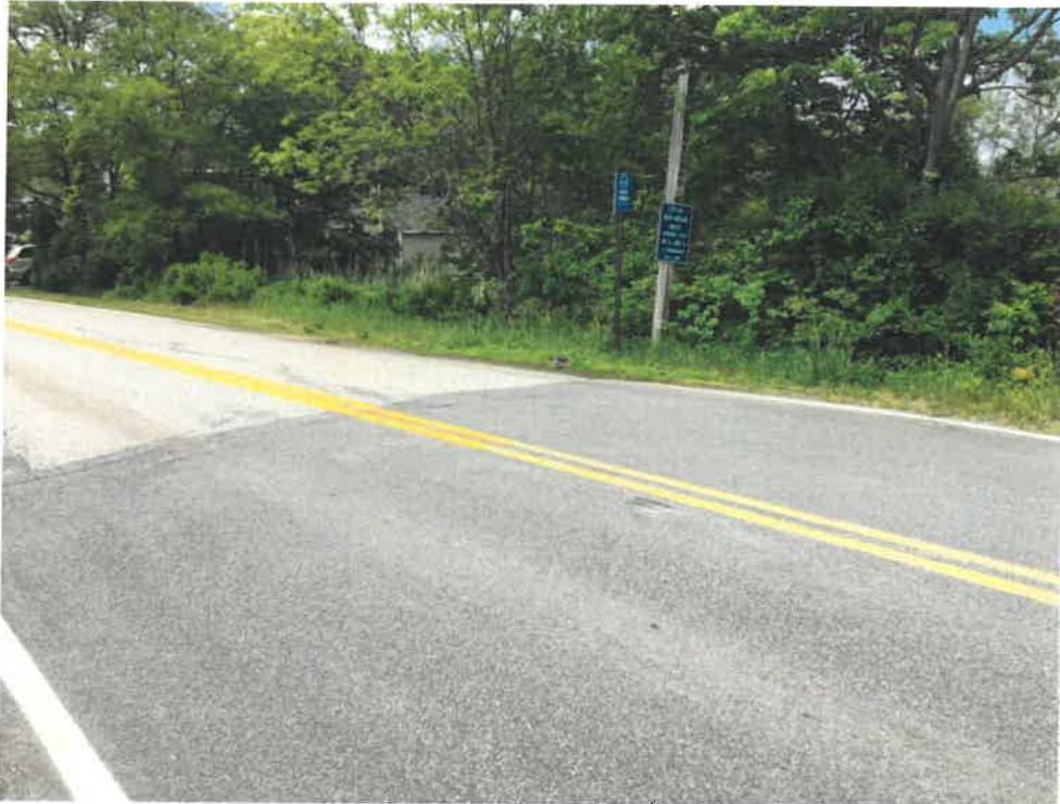
Photo 1 (06-06-18): Facing northeasterly at Spurwink Avenue crossing with Trout Brook which is an Urban Impaired Stream. Culvert crossing coincides with the pavement crack and change in pavement seam (which is also the South Portland municipal boundary) across the surface of Spurwink Avenue. Smaller blue sign indicates that the culvert is in the Trout Brook Watershed.
