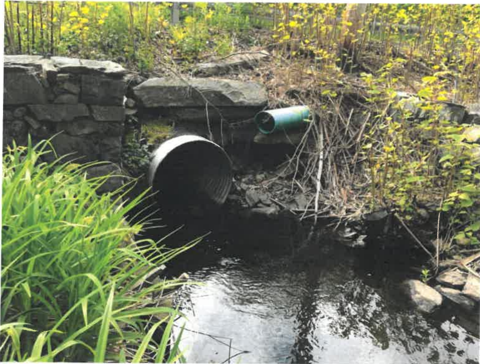
Photo 7 (06-06-18): Submerged outlet of culvert on the east side of Shore Road. Loose stones on headwall of outlet with smaller diameter green polyvinylchloride (pvc) pipe discharging well above the outlet invert elevation of the cross culvert.
