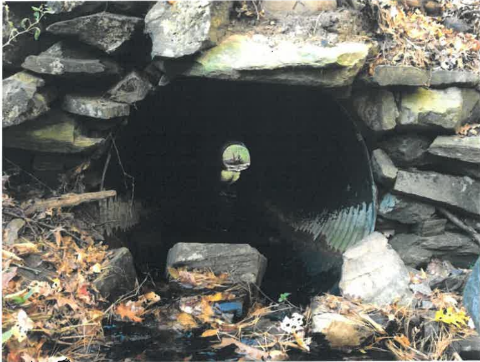
Photos 3 (10-22-18): Looking through the culvert from the inlet side, interior of the pipe appears visually to be in a degraded condition with the invert of the pipe clearly corroded.
