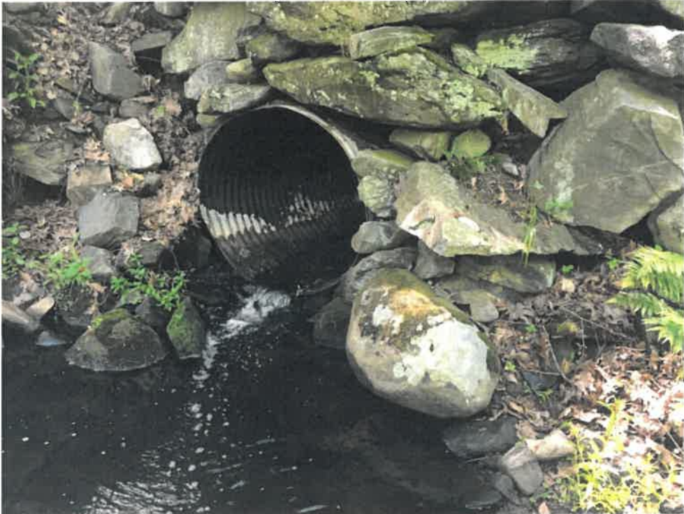
Photo 6 (06-06-18): Hanging outlet of the aluminum elliptical pipe with flared end and rip rap headwall. Additional rip rap would be desirable to bolster the area around the culvert.
