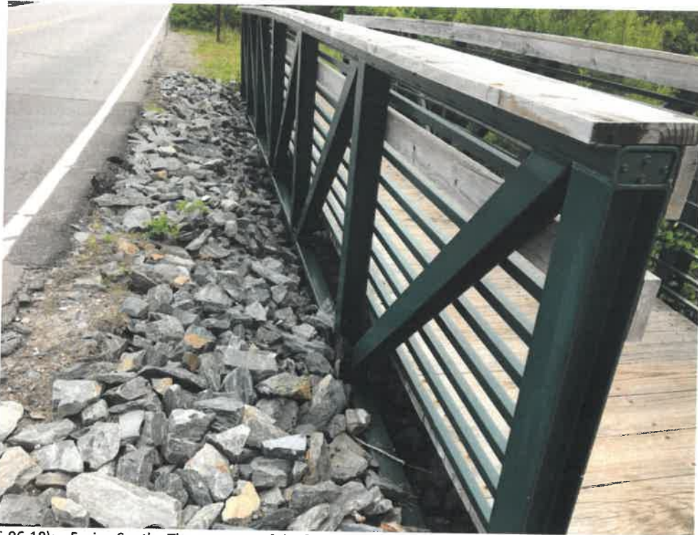
Photo 3 (06-06-18): Facing South. The presence of the footbridge directly over the culvert inlets and stone rip rap make inlet maintenance a challenge
