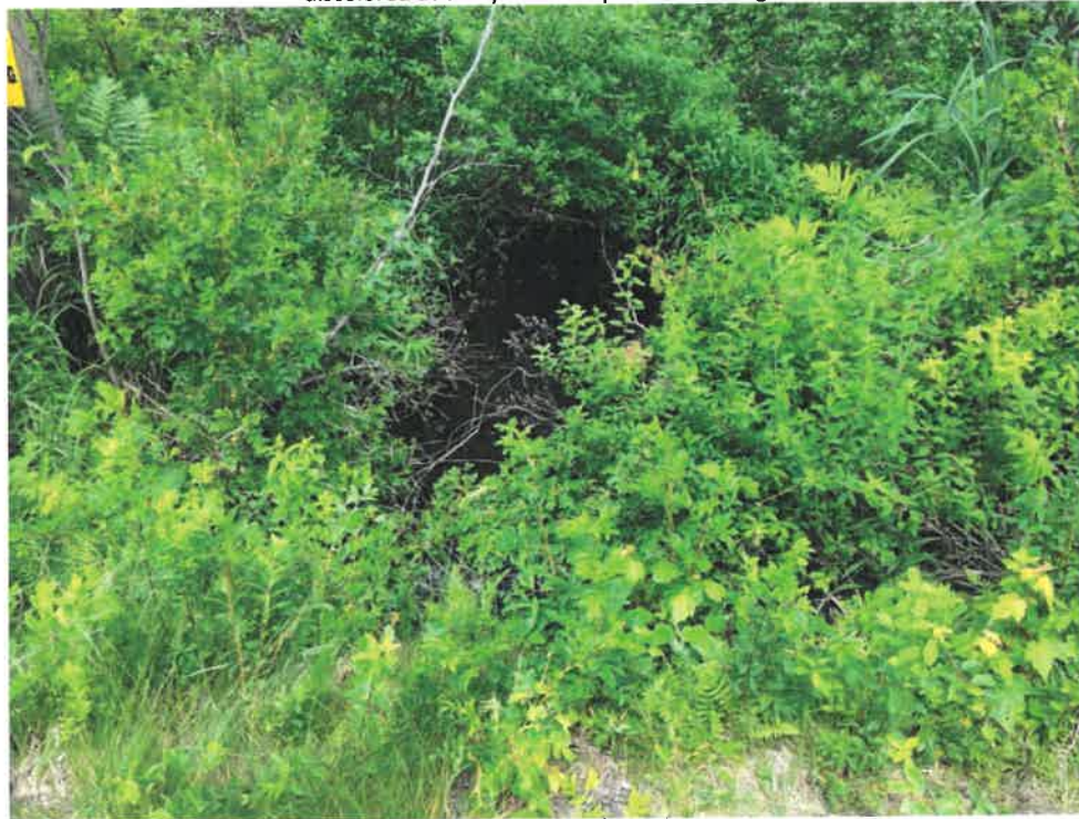
Photo 6 (06-20-18): Facing northeast at the downstream channel of the culvert outlet. Thick vegetation and likely deposited sediment within the channel create standing water with a very slow flow rate.
