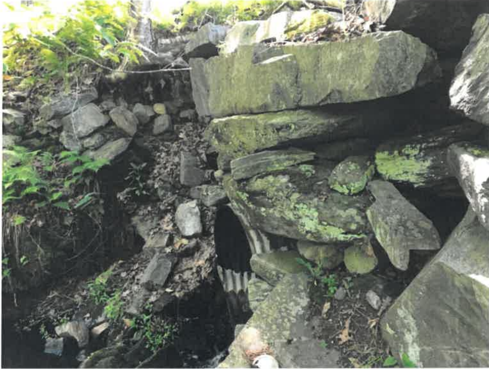
Photo 7 (06-06-18): Stone headwall at the outlet has deteriorated and has many loose and dislodged stones.
