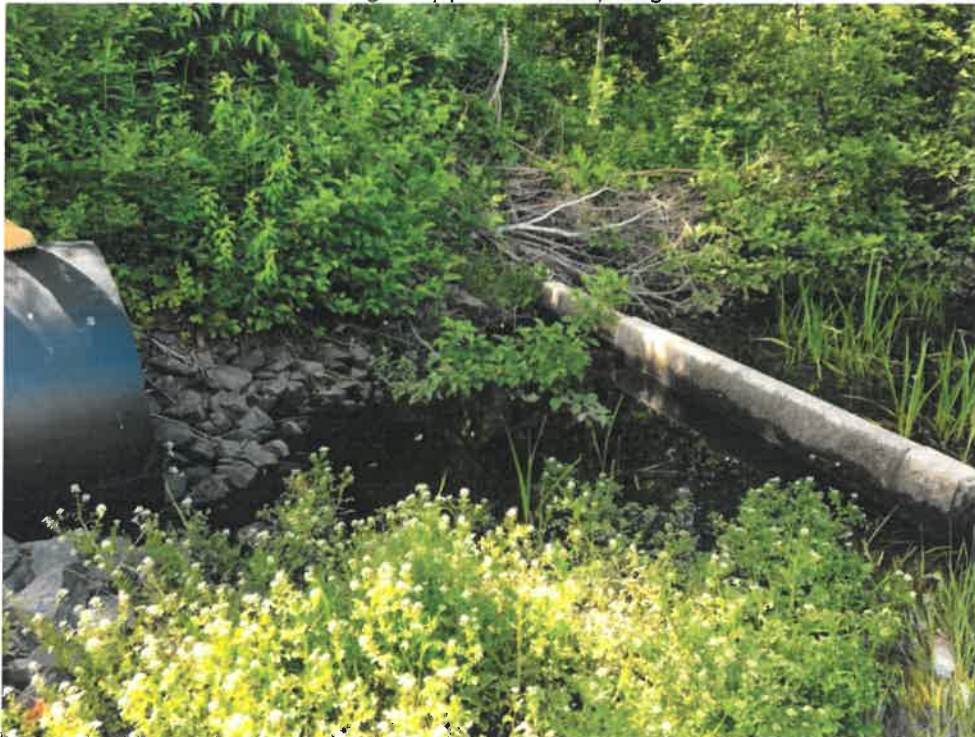
Photo 6 (06-20-18): Outlet of culverts on the east side of Old Ocean House Road. Outlet has a rip rap lined plunge pool and headwall. Concrete weir at outlet was installed to create a submerged outlet to allow alewife fish passage.
