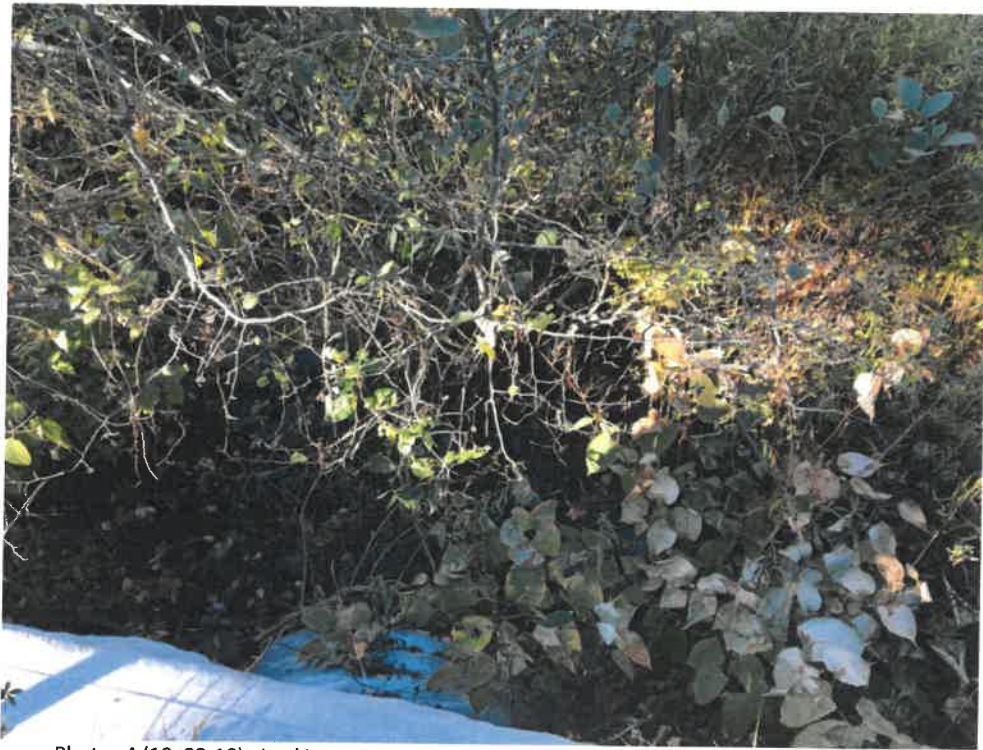
Photos 4 (10=22-18): Looking west at an overhead view of the inlet of culvert on Shore Road.
