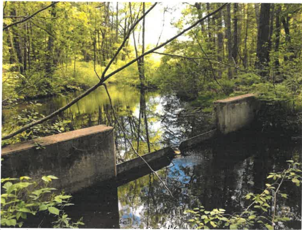
Photo 6 (06-06-18): Impoundment area with concrete and steel wall with a v-notch weir remotely located upstream of the Shore Road culvert. Two impoundments flow in series and then combine with the outflow from the nearby Dyer Pond Road culvert to discharge into the Shore Road culvert.
