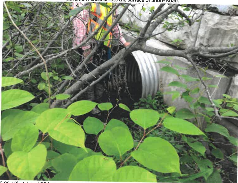
Photo 2 (06-06-18): Inlet of 36-inch corrugated aluminum cross pipe with a cast-in-place concrete collar and base set within a large concrete block "Stonestrong" retaining wall. Inlet is on the west side of Shore Road.
