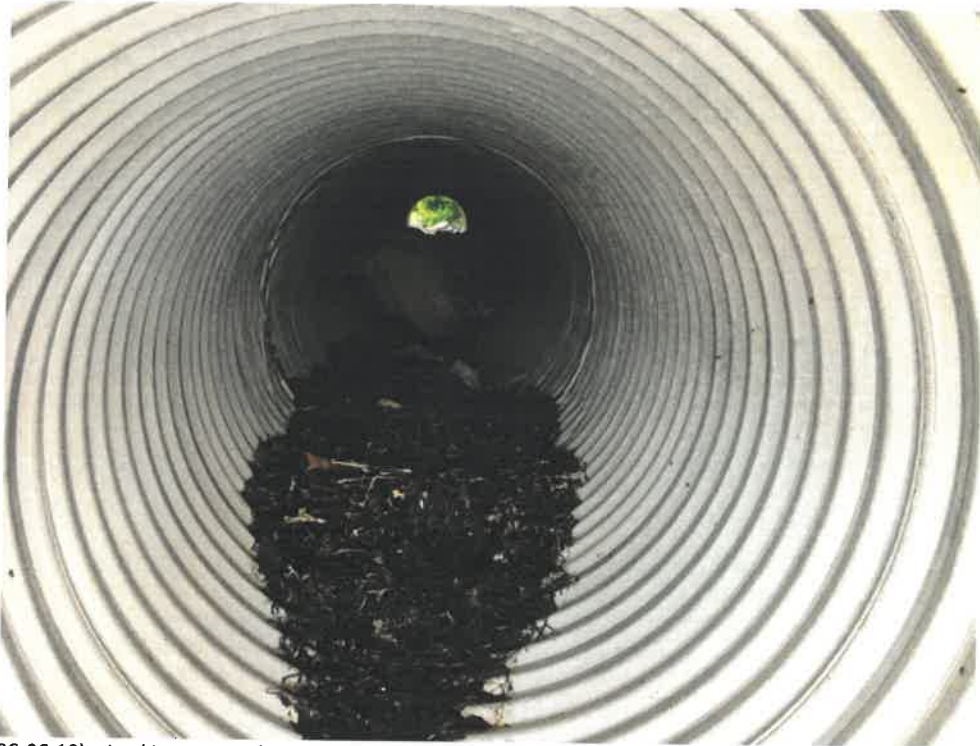
Photo 7 (06-06-18): Looking west at large rock and other ocean debris inside of northerly culvert. Being exposed directly to Casco Bay, ocean surges often push debris inside of these pipes creating an ongoing maintenance issue for the Town.
