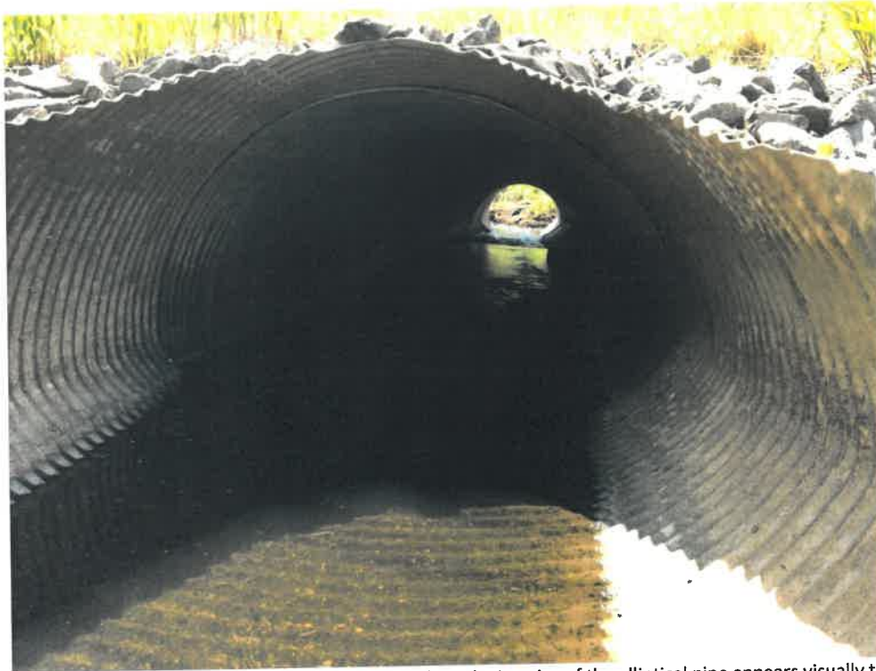
Photos 3 (06-06-18): Looking through the culvert from the inlet side, interior of the elliptical pipe appears visually to be in good condition, however, the flared end section appears to be pulling away from the last section of pipe.
