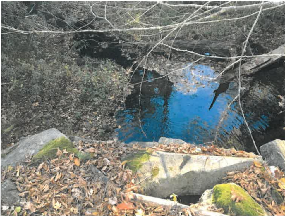
Photo 8 (10-22-18): Overhead view of culvert outlet with loose stones in the stone headwall.
