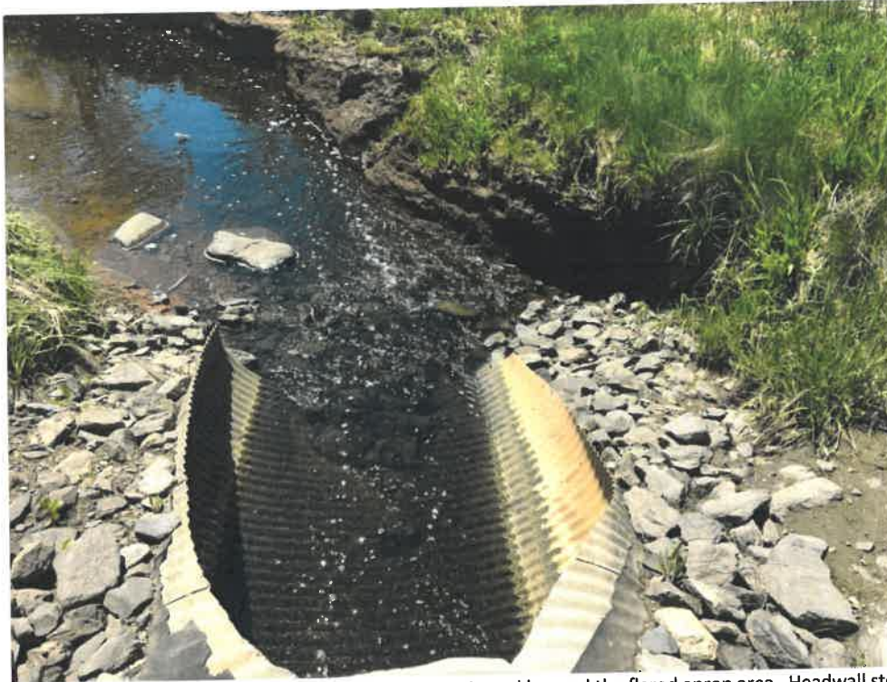
Photo 7 (06-06-18): Overhead view of culvert outlet with stones in and beyond the flared apron area. Headwall stones around the culvert appear to be depleted of rip rap layers and should be replenished.
