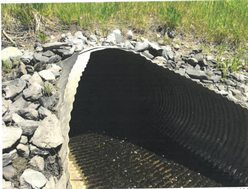
Photo 5 (06-06-18): Submerged outlet of the aluminum elliptical pipe with flared end and rip rap headwall. Additional rip rap would be desirable to bolster the area around the culvert.
