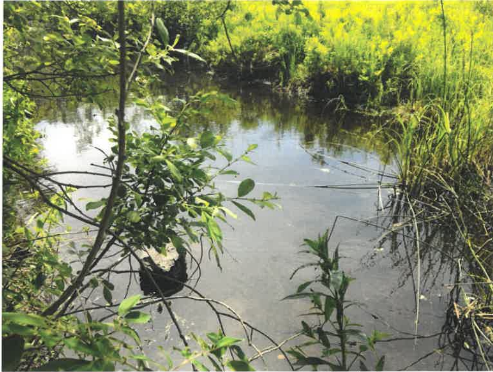
Photos 3 (06-20-18): Looking upstream at the Alewife Brook flow to the Inlet of the culvert on west side of Ocean House Road (Route 77). Alewife Brook hydraulically connects Great Pond to Casco Bay.
