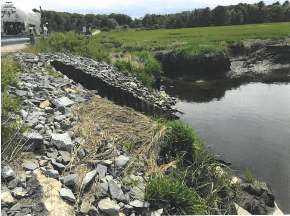
Photo 5 (06-06-18): Submerged outlet of the aluminum elliptical pipe with flared end and rip rap headwall on the west side of Sawyer Road. Quantity of rip rap appears to be sufficient on the outlet area around the culvert.
