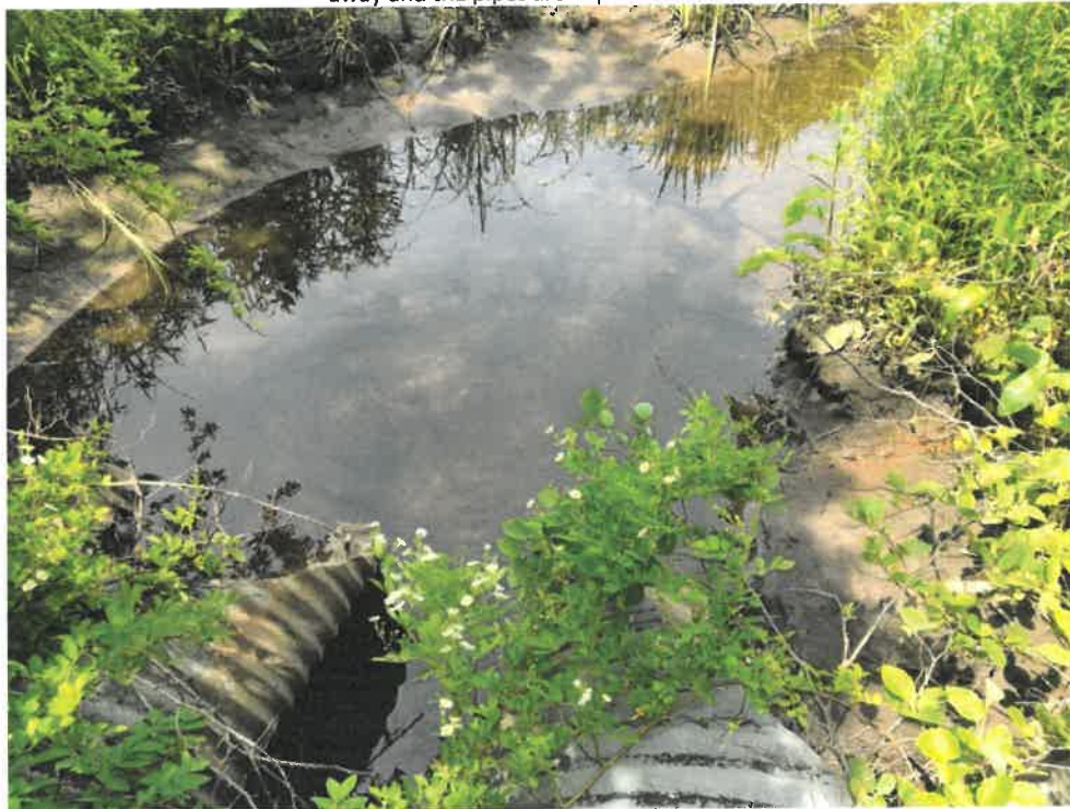
Photos 4 (06-20-18): Looking down from onto one the two culverts' inlets. Culverts' inlet area is wide just upstream from the pipes with a narrower channel further upstream flowing toward the culverts.
