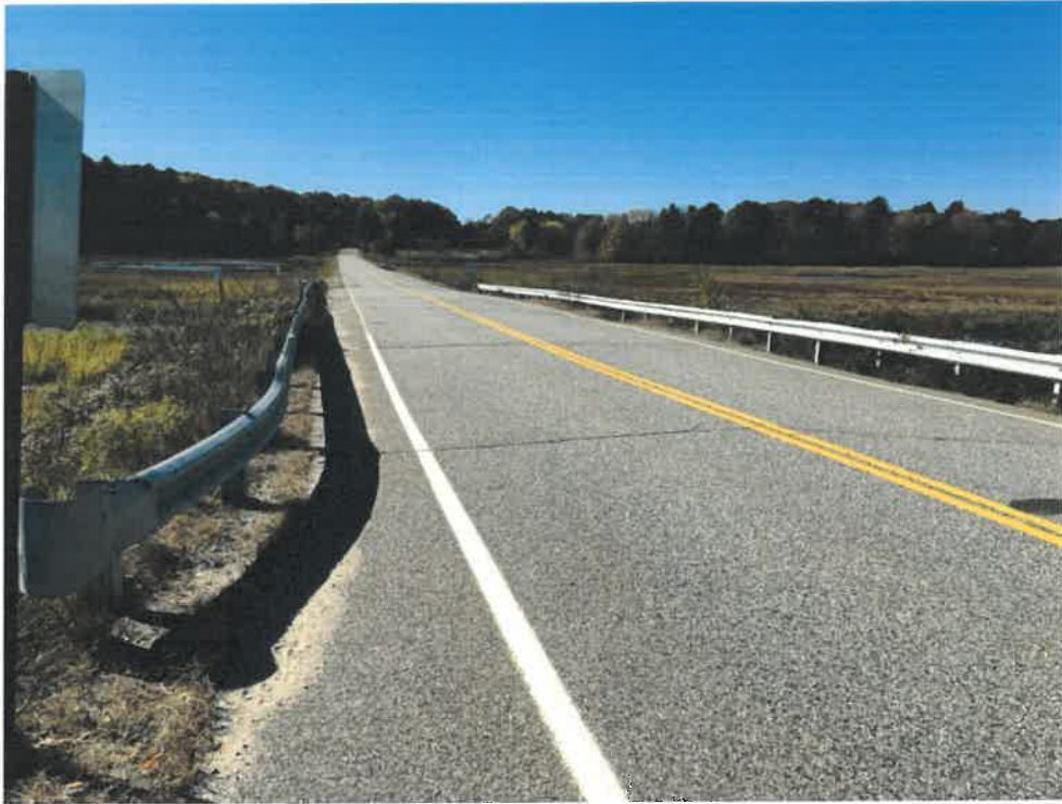
Photo 1 (10-22-18): Facing southwest at Sawyer Road culvert crossing. Road routinely floods beyond culvert crossing at low area of roadway elevation.
