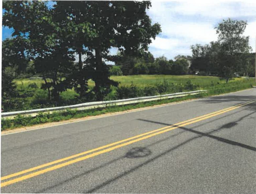
Photo 1 (06-20-18): Facing southeast at Old Ocean House Road crossing of Alewife Brook. Culvert are located relatively deep in relation to the road surface elevation with a steep roadway embankment.
