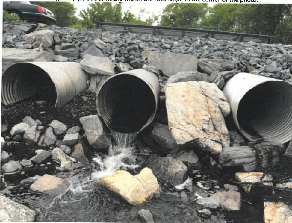
Photo 6 (06-06-18): Looking east at hanging outlet of the three, 36-inch aluminum corrugated pipe outlets on the west side of Shore Road. Seaweed and other debris frequently compromise the culverts' capacity as exemplified by only the center culvert flowing freely despite all three culverts being installed at roughly the same elevations.
