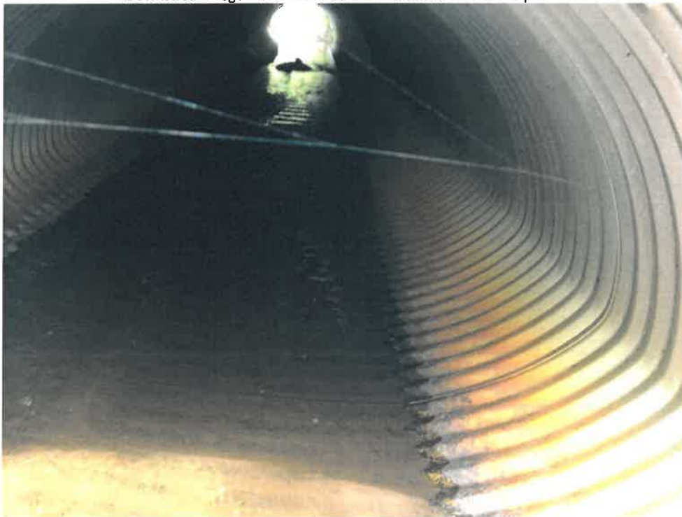
Photo 6 (06-06-18): Interior view of culvert taken from outlet to the inlet of culvert. Some corrosion visible along invert of pipe, however, the culvert appears visibly to be in good condition.
