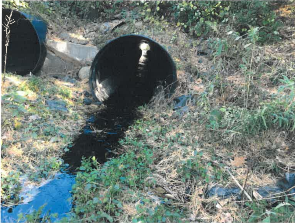
Photo 3 (10-22-18): Looking northerly through the inlet of one of the two 48-inch high density polyethylene liner pipes within the original corrugated aluminum cross pipes. The invert of the main carrying pipe is lined with a corrugated metal pipe section to reduce the velocity of flow through the pipe.
