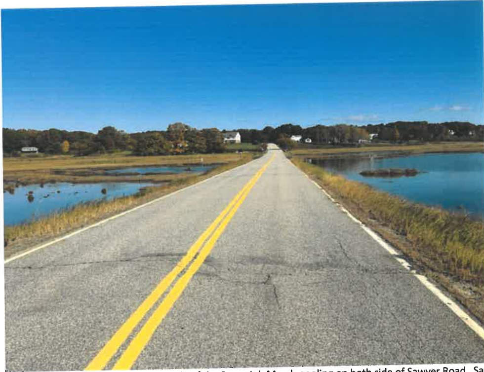
Photo 9 (10-22-18): Facing north during high tide of the Spurwink Marsh pooling on both side of Sawyer Road. Sawyer Road floods often during intense weather and tide events in the foreground of the photo as the road elevation is lower than at the culvert crossing which the inlet to the Spurwink River culvert is visible on the right side (east) of Sawyer Road.
