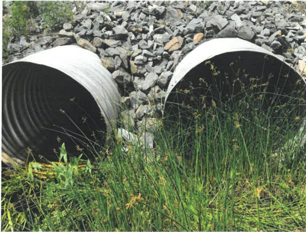
Photo 5 (06-20-18): Outlet of culverts on the south side of Scott Dyer Road. Westerly (left) pipe is set lower and carries the primary flow. Easterly culvert is partially blocked by vegetation.
