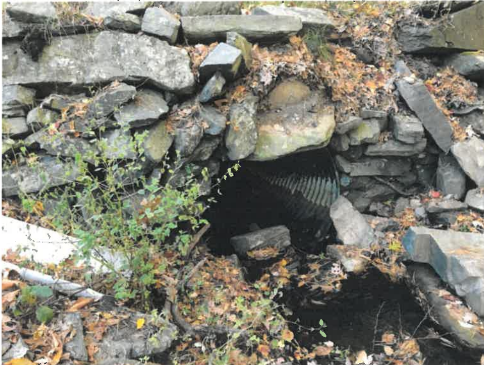
Photo 2 (10-22-18): Submerged inlet of 48-inch corrugated metal pipe with corroded invert and various stones blocking the inlet from reaching full flow capacity. The stone headwall needs to be reset.
