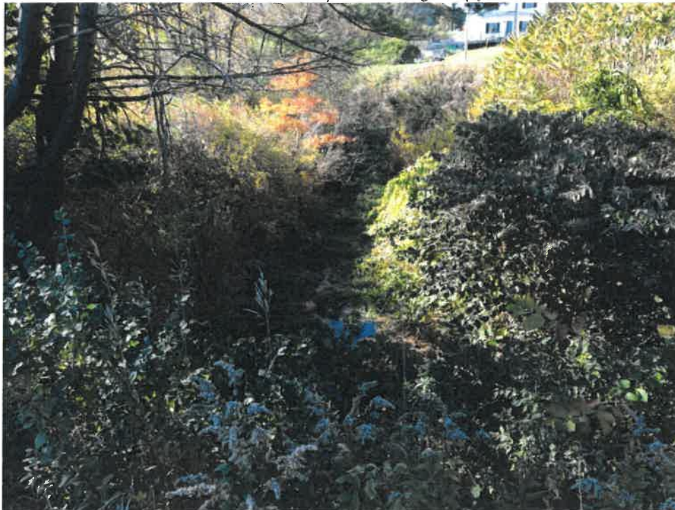
Photos 4 (10-22-18): Looking northwesterly from top of embankment at the upstream channel flowing to the two culverts inlets on the west side of Old Ocean House Road.
