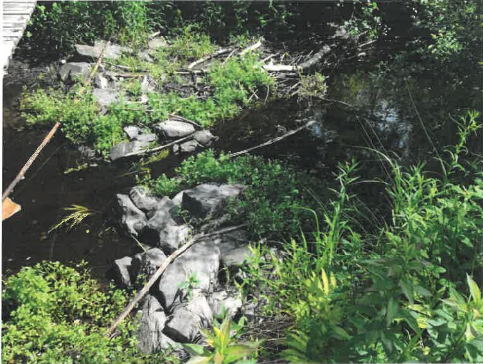
Photo 7 (06-20-18): Downstream channel of the culvert outlet flow with stone weir wall with center opening to control elevation and flow from the culverts to dissipate energy of the outfall and reduce the velocity of the outflow to the receiving channel. The weir also creates a pool area within the channel.
