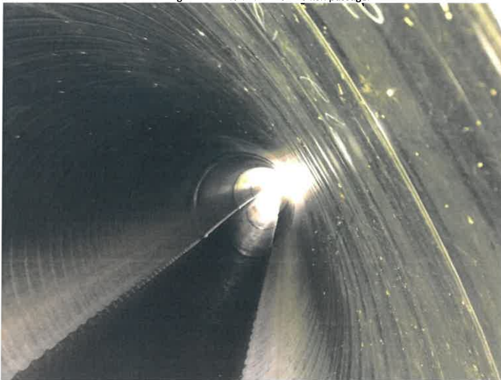
Photo 6 (06-20-18): View of the interior of the HDPE liner from the outlet toward the inlet of the pipe. Invert of the culvert is submerged.
