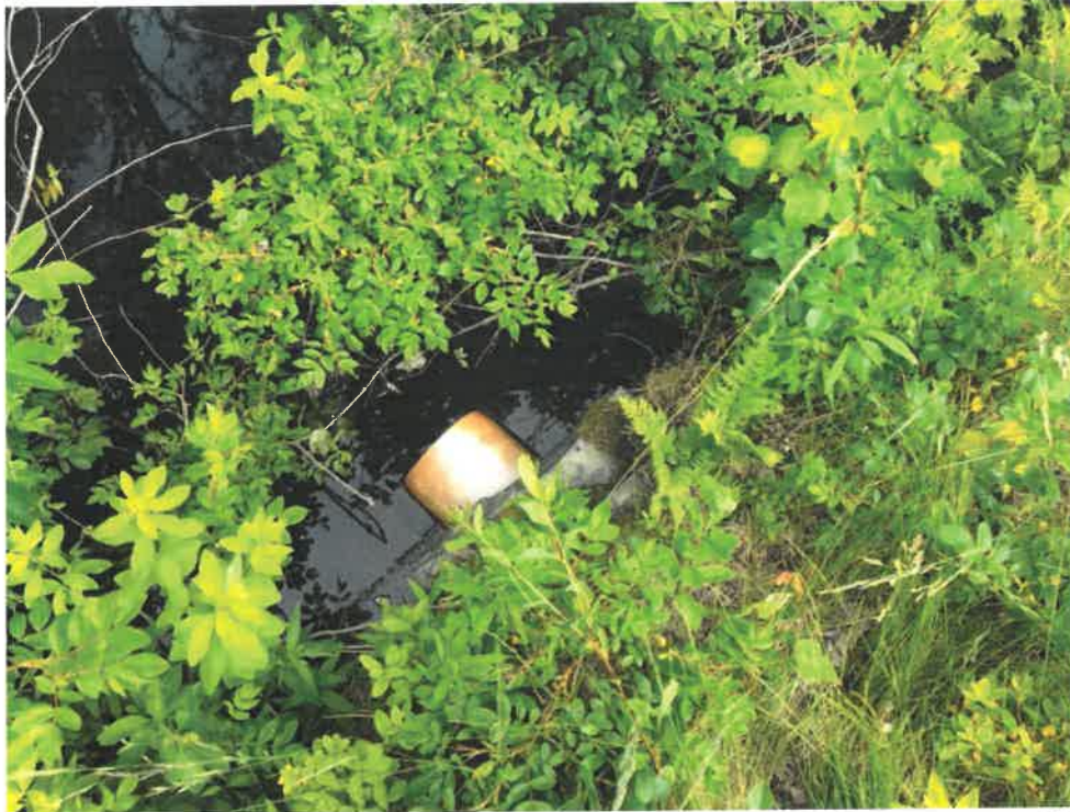
Photo 5 (06-20-18): Overhead view of submerged culvert outlet with a stone placed over the pipe to act as a headwall. Pipe is discolored due to years of exposure to sunlight.
