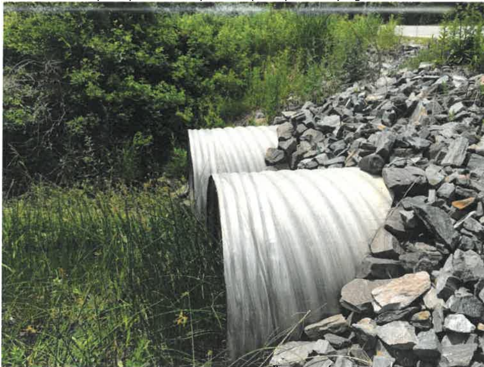
Photo 6 (06-20-18): Culvert outlet discharge of Willow Brook on the south side of Scott Dyer Road. Some limited vegetation removal and rip rap at the end of the easterly pipe would ensure that its capacity is not compromised by additional vegetation growth.
