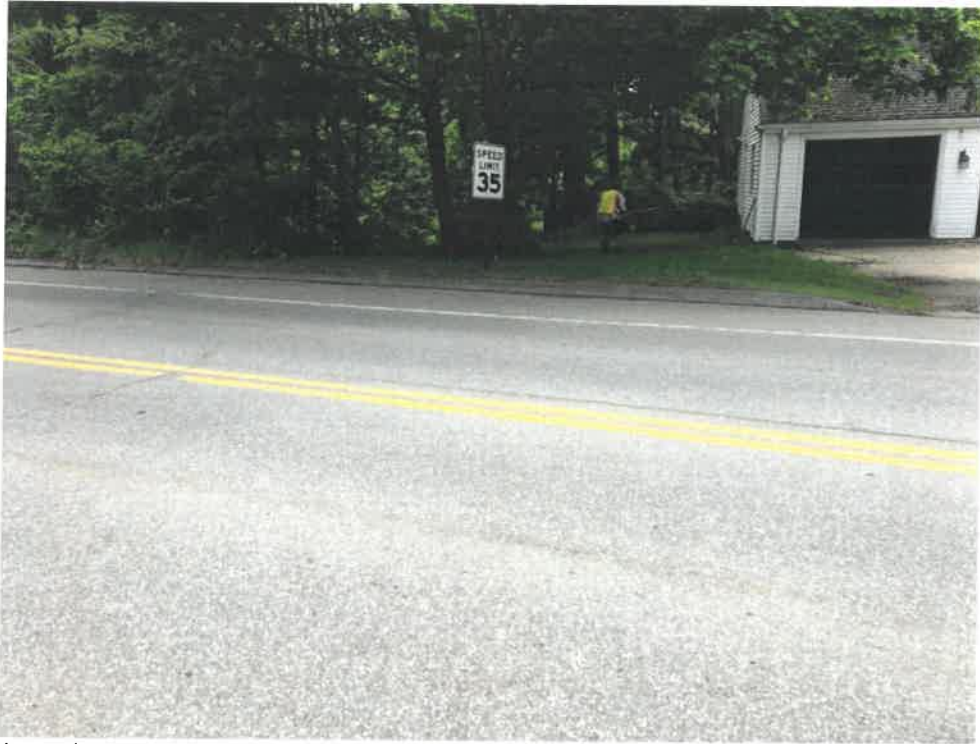
Photo 1 (06-06-18): Facing northeast at Ocean House Road (Route 77) crossing of the Trout Brook culvert.
