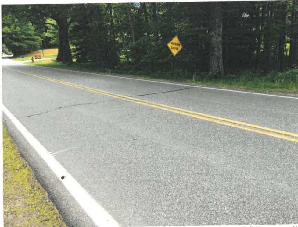
Photo 1 (06-06-18): Facing south at pavement surface of the Spurwink Avenue culvert crossing for an unnamed tributary to Trout Brook. Culvert crossing coincides with the pavement crack across the surface of Spurwink Avenue in the center of photo.
