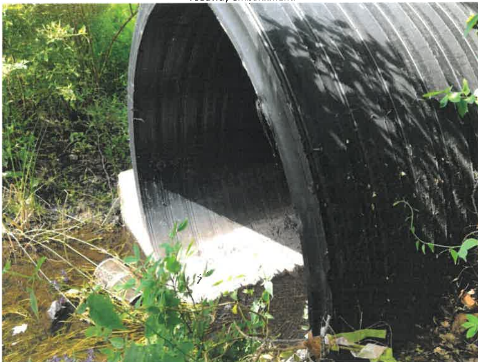
Photo 2 (06-20-18): Submerged inlet of the 70-inch high density polyethylene liner pipe within the original corrugated aluminum cross pipe. Pipe is supported on a concrete saddle.
