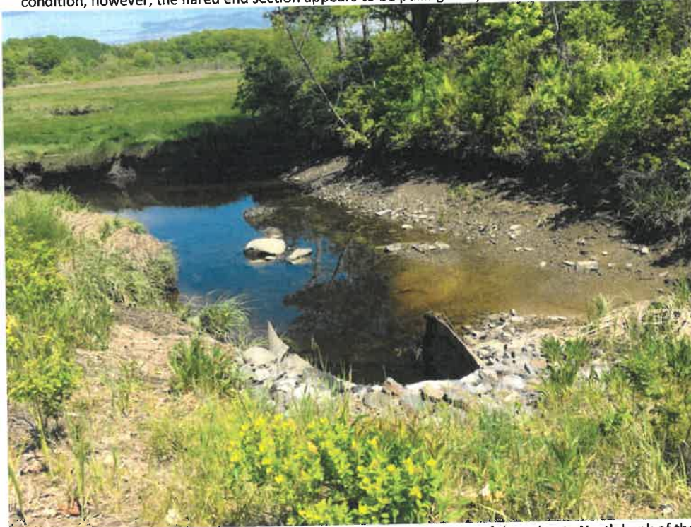
Photo 4 (06-06-18): Inlet to culvert with channel of the Spurwink River upstream of the culvert. North bank of the channel is eroded due to the sharp bend in channel just upstream of the culvert location and may need to be bolstered with rip rap armor at some point in the future.
