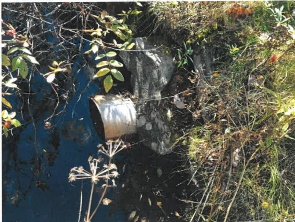
Photo 4 (10-22-18): Submerged outlet of culvert on the east side of Eastman Road. No rip rap apron has been provided. Area around the outlet has thick vegetation and standing water and is not draining well.
