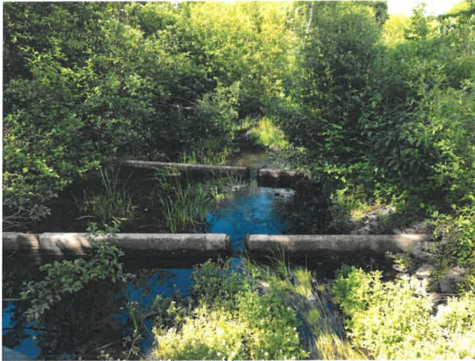
Photo 7 (06-20-18): Downstream channel of the culvert outlet flow with two concrete weir walls with slotted weirs to control elevation and flow from the culverts to dissipates energy of the outfall and reduce the velocity of the outflow to the receiving channel. The weirs also create pool areas within the channel.
