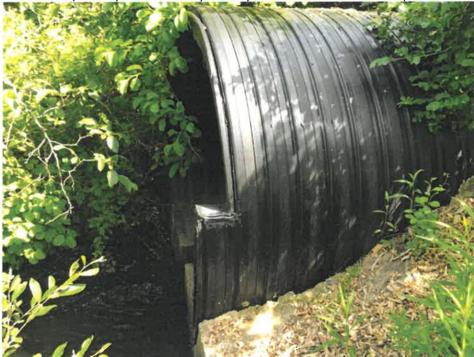
Photo 4 (06-20-18): Submerged outlet of culvert with slotted weir invert to slow the flow velocity through the pipe to allow fish passage. Culvert outlet is supported by concrete saddle.
