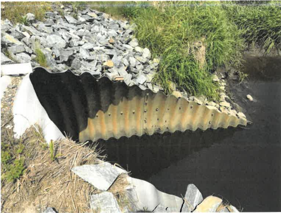
Photo 2 (06-20-18): Submerged inlet of 10.5-foot wide by 11.5-foot tall corrugated aluminum elliptical pipe with flared end and rip rap headwall on east side of Sawyer Road. Additional headwall rip rap should be added to the headwall.
