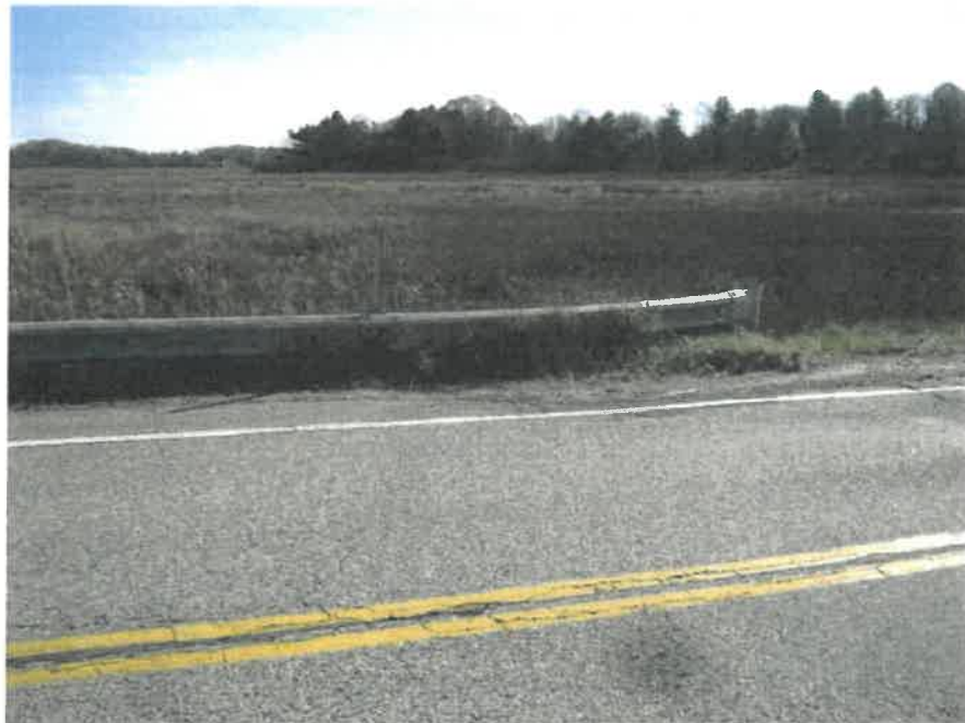
PHOTO 6 Description View showing low approach rail
