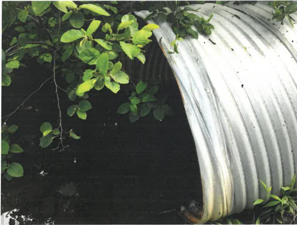
Photo 5 (06-06-18): Culvert outlet on east side of Spurwink Avenue is submerged within the corrugated aluminum pipe. Downstream vegetation obscured channel at the time of the photo.
