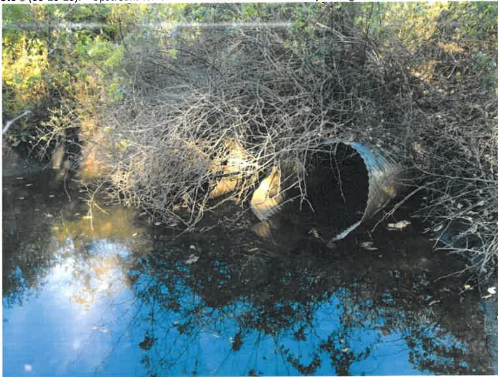
Photo 6 (10-22-18): One of the outlets of the culverts on the south side of the embankment is obscured by vegetation and partially buried in sediment. Outlet has some stone in the channel, but no formal plunge pool or visible headwall.
