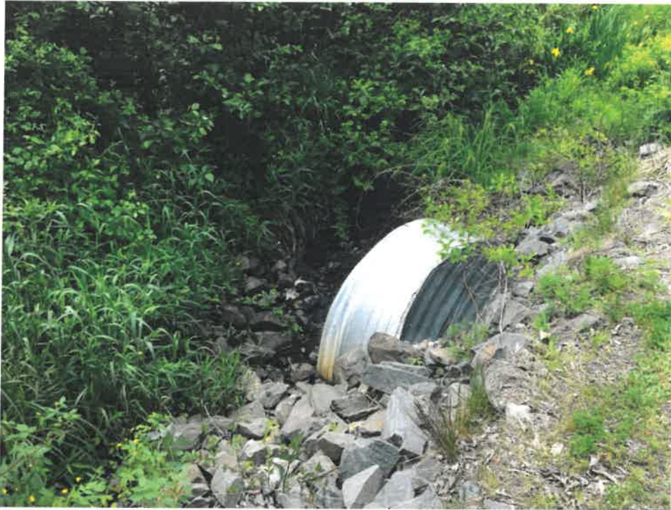
Photos 3 (06-06-18): Culvert inlet on west side of Spurwink Avenue is submerged within the corrugated aluminum pipe. Upstream vegetation obscured channel at the time of the photo.
