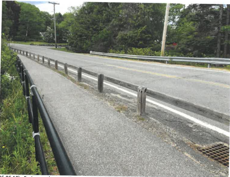
Photo 1 (06-06-18): Facing northeast at Shore Road crossing of the Dyer Pond outflow. Culvert crossing coincides with the pavement crack across the surface of Shore Road.
