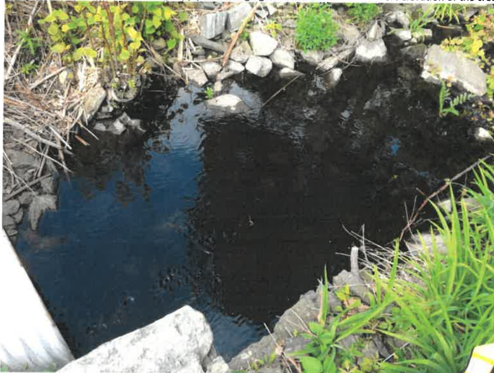
Photo 8 (06-06-18): Overhead view of culvert outlet with rip rap plunge pool apron area. Stone lined plunge pool dissipates energy of the outfall and reduces the velocity of the outflow to the receiving channel.
