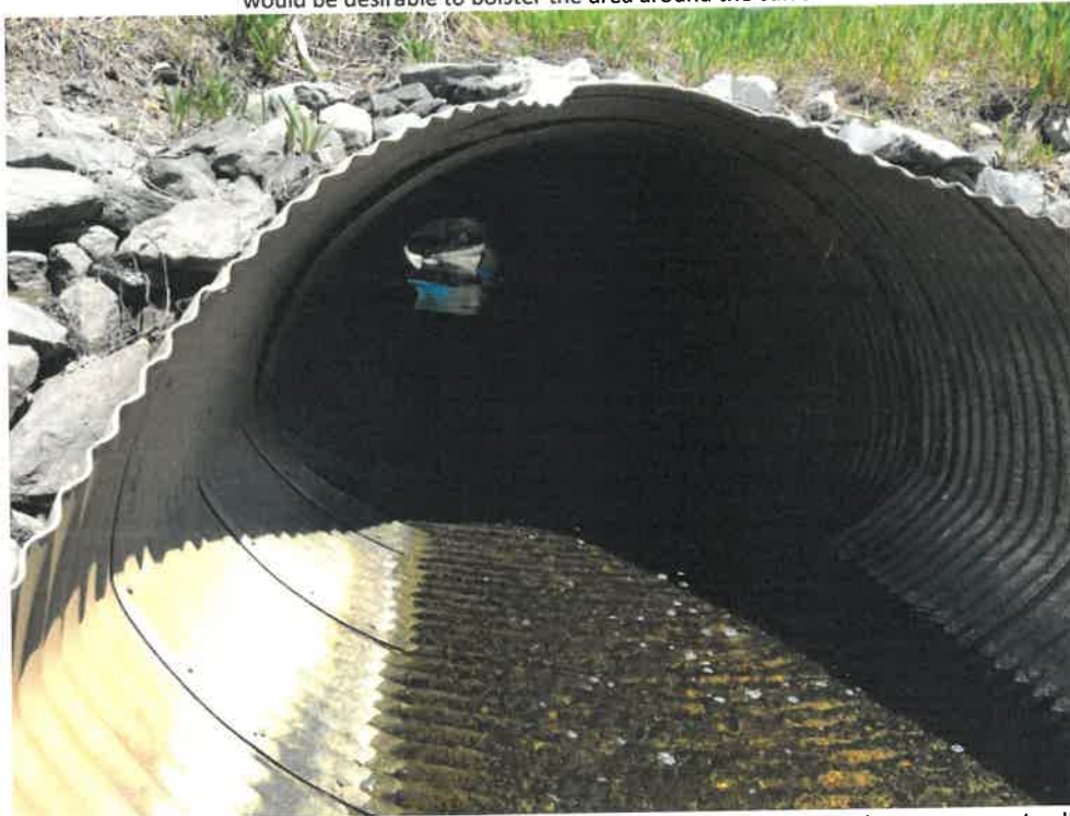
Photo 6 (06-06-18): Looking through the culvert from the outlet side, interior of the elliptical pipe appears visually to be in good condition, however, the flared end section appears to be pulling away from the last section of pipe.
