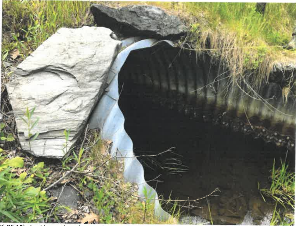
Photo 6 (06-06-18): Looking at the submerged outlet of 8 foot, 2-inch-wide by 5 foot, 9-inch-high steel plate pipe arch cross pipe. Rip rap stones are sparse, but provide a headwall.
