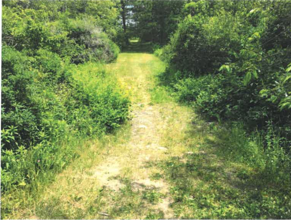
Photo 1 (06-20-18): Facing east at the Sanitary Sewer Embankment crossing which also acts as a recreational trail connection to the Town Center. Culverts are located relatively deep in relation to the top elevation of the embankment. Stones visible in cleared area is the location of the emergency spillway.
