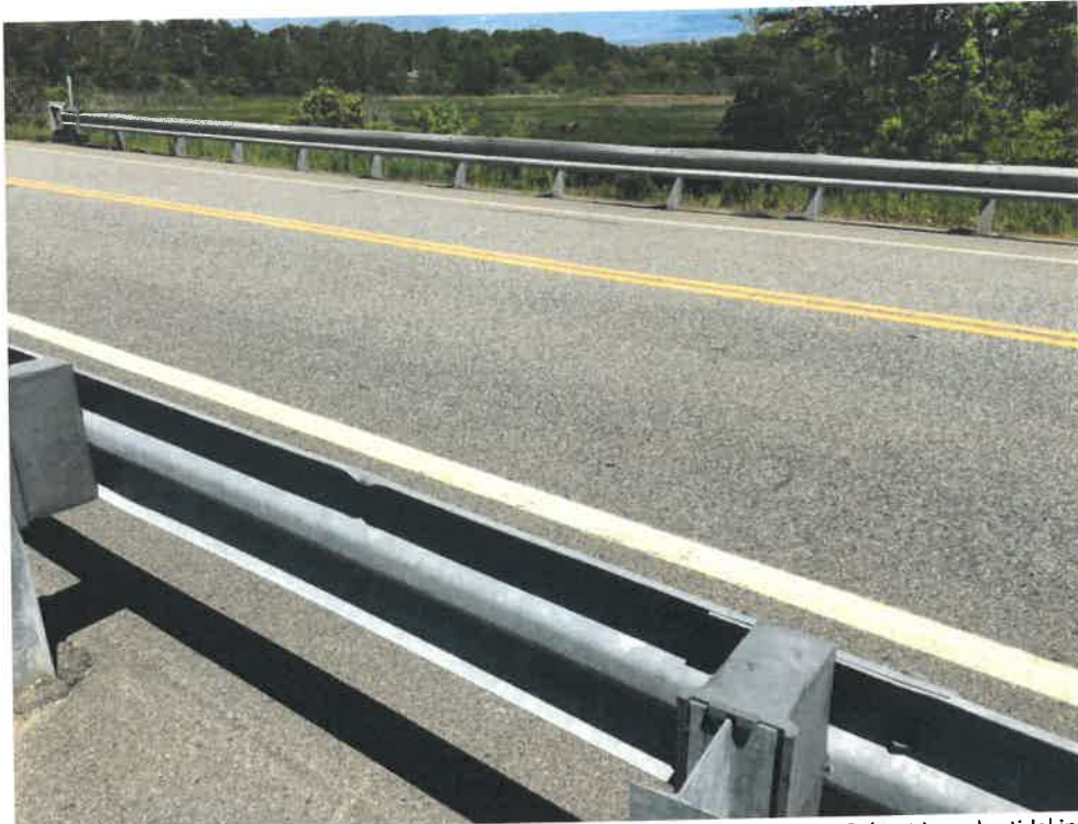
Photo 1 (06-06-18): Facing southwest at Spurwink Avenue crossing of the Spurwink River. Culvert is under tidal influence and the Spurwink Marsh is in the background.
