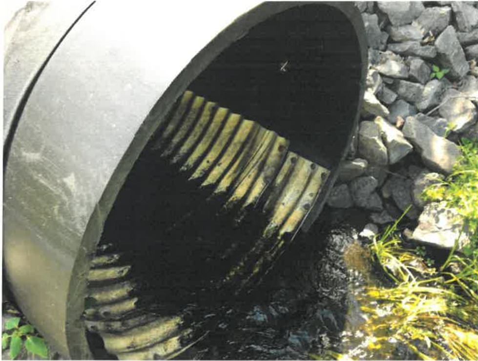
Photo 5 (06-20-18): Submerged outlet of main flow carrying culvert with corrugated metal pipe invert to slow the flow velocity through the pipe to allow fish passage.
