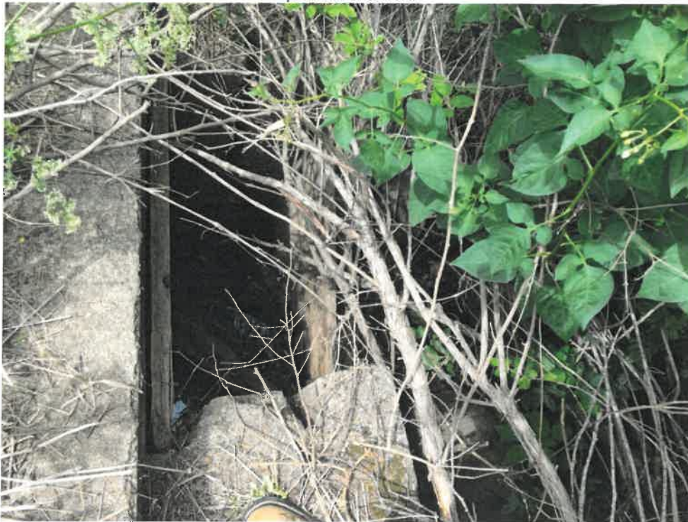
Photo 2 (06-20-18): Inlet of 36-inch High Density Polyethylene (HDPE) pipe headwall on northeast side of Sawyer Road. Concrete headwall conceals the HDPE pipe and pieces of concrete support wooden boards that creates an inlet weir to create an impoundment upstream of the pipe.
