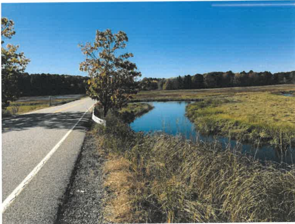
Photo 8 (10-22-18): Facing south during high tide of the Spurwink River on the outlet to the west of Sawyer Road. The Spurwink River channel downstream of culvert outlet flows through a wide pool area before flowing north parallel with Sawyer Road before turning to the west and winding toward the Atlantic Ocean.
