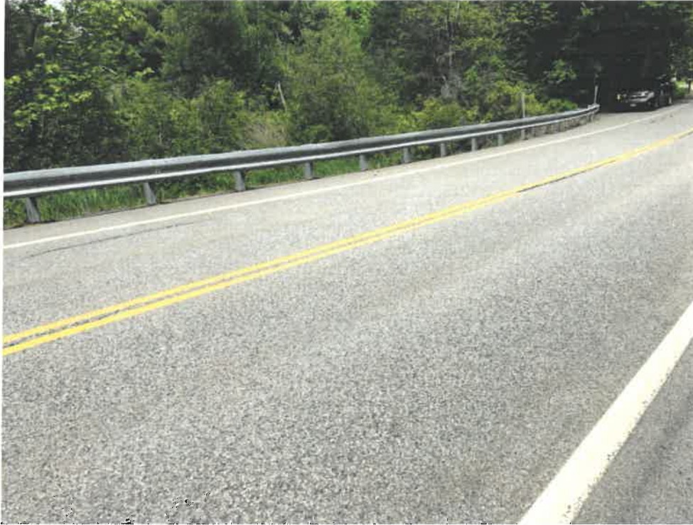
Photo 1 (06-06-18): Facing north at the surface of Spurwink Avenue at the crossing of the pond outlet pipe/culvert that discharges into Pollack Brook.
