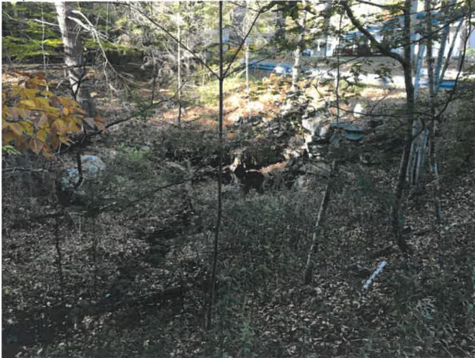
Photo 10 (10-22-18): Facing south from the nearby pump station at the downstream flow of Pond Cove Brook from the Mitchell culvert outlet.
