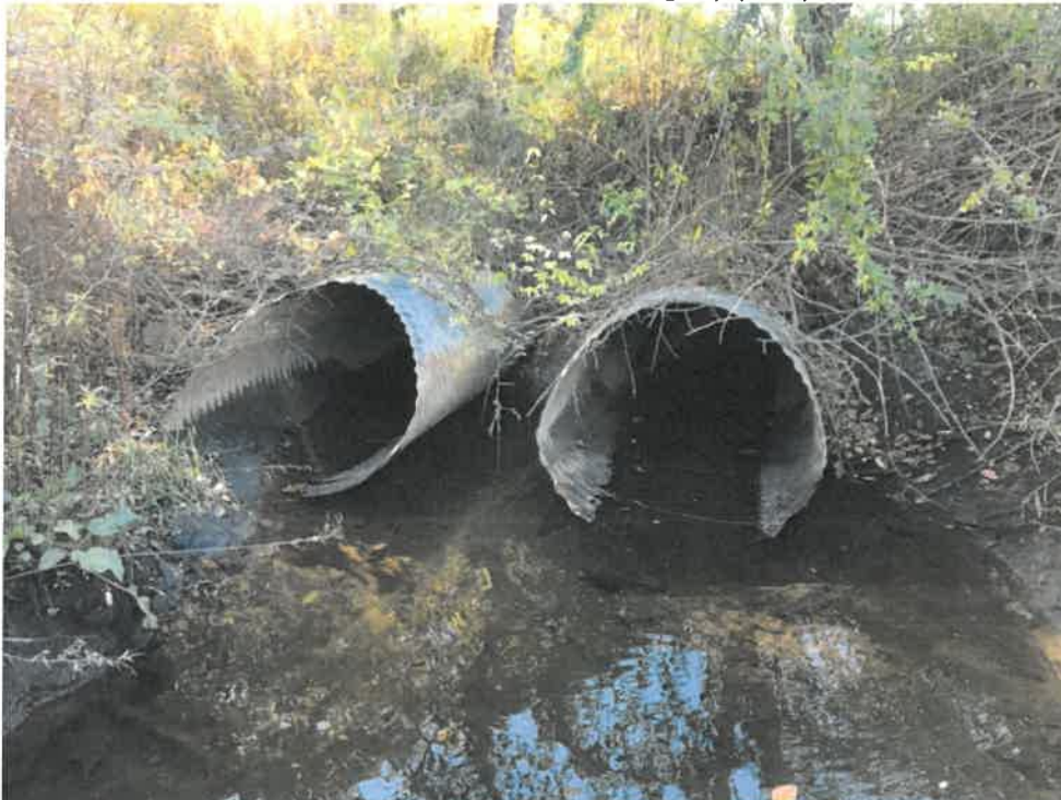
Photo 2 (10-22-18): Inlets of the two, 48-inch wide by 36-inch tall corrugated aluminum pipes located northerly of the sanitary sewer crossing embankment. Inverts to both pipes are corroded and in decay.
