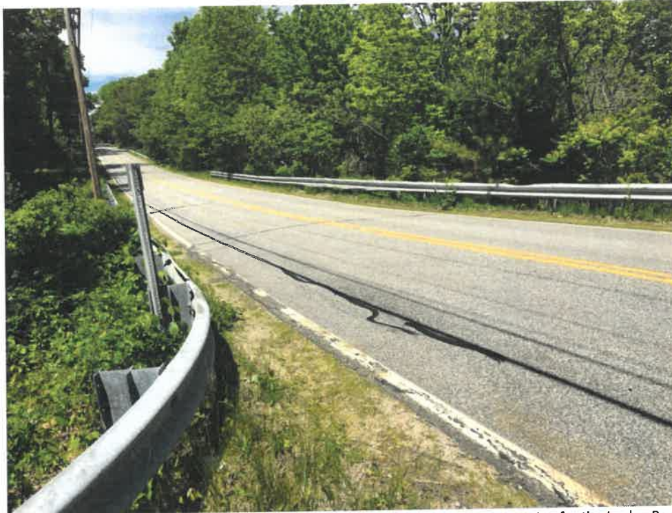
Photo 1 (06-06-18): Facing north at pavement surface of the Spurwink Avenue culvert crossing for the Jordan Pond outflow. Culvert crossing coincides with the pavement crack across the surface of Spurwink Avenue in the center of photo.
