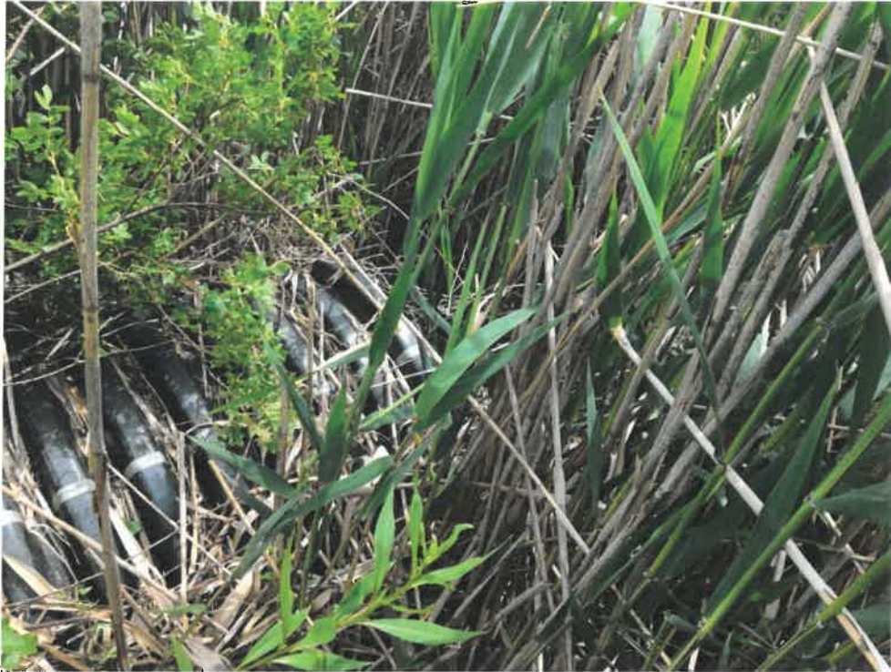
Photo 5 (06-06-18): Submerged outlet of the HDPE pipe on the west side of Sawyer Road. Thick vegetation around the end of the culvert could be better controlled with a rip rap apron.
