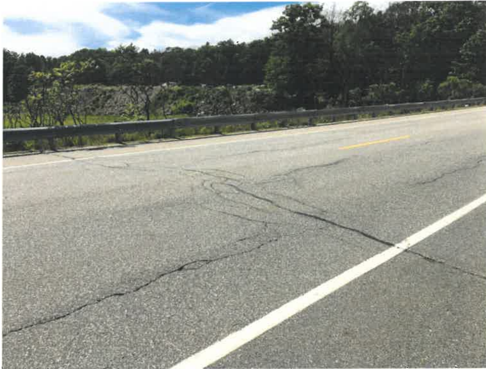
Photo 1 (06-20-18): Facing west at Ocean House Road (Route 77) crossing of Alewife Brook. Culvert location coincides with the crack across the pavement surface. Culvert is located relatively deep in relation to the road surface elevation with a steep roadway embankment.
