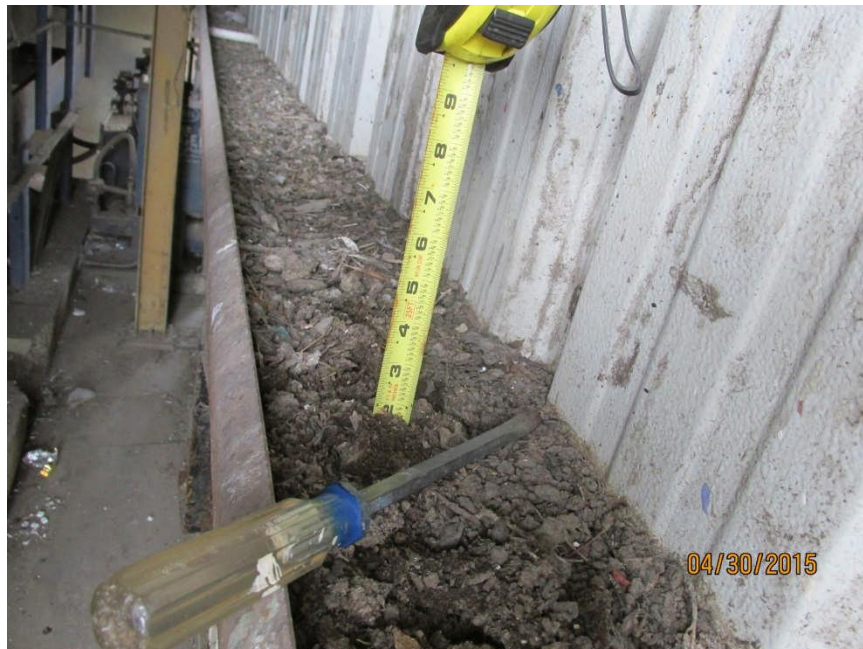
Photo #6 – Lower Level East Wall of Building: horizontal Z-girt with over 2" of continuous soil/debris.
