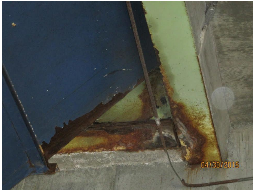
Photo #8 – Lower Level Hopper & Floor Beams (Above): corrosion of painted hopper and steel floor beams.
