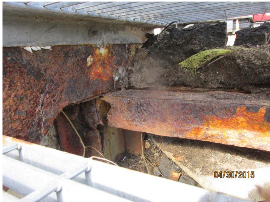
Photo #10 – Exterior Stair on North Side: heavy corrosion of angle bracket below top landing.
