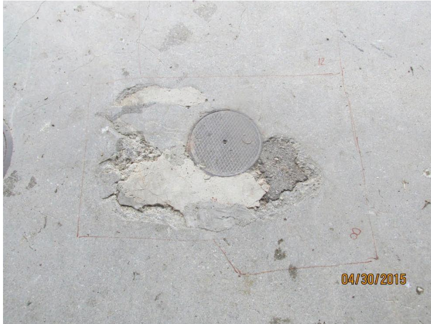
Photo #3 – Upper Level Hopper Slab: typical area with concrete spalling.
