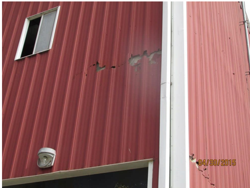
Photo #4 – Southeast corner of building: typical holes rusted through metal wall panels.
