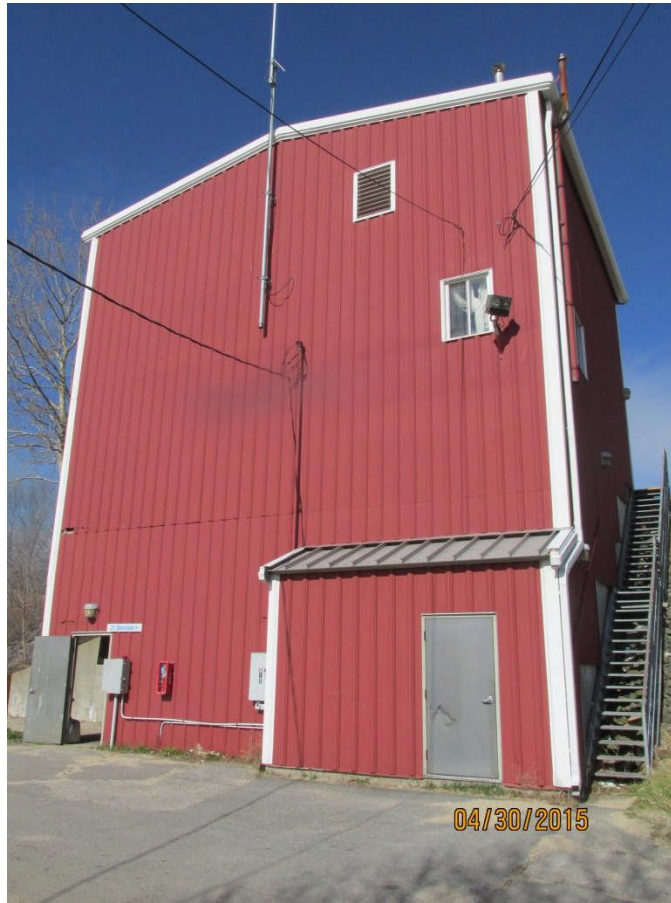
Photo #5 – East Elevation of Building: wall panels extend to grade on left side of photo.
