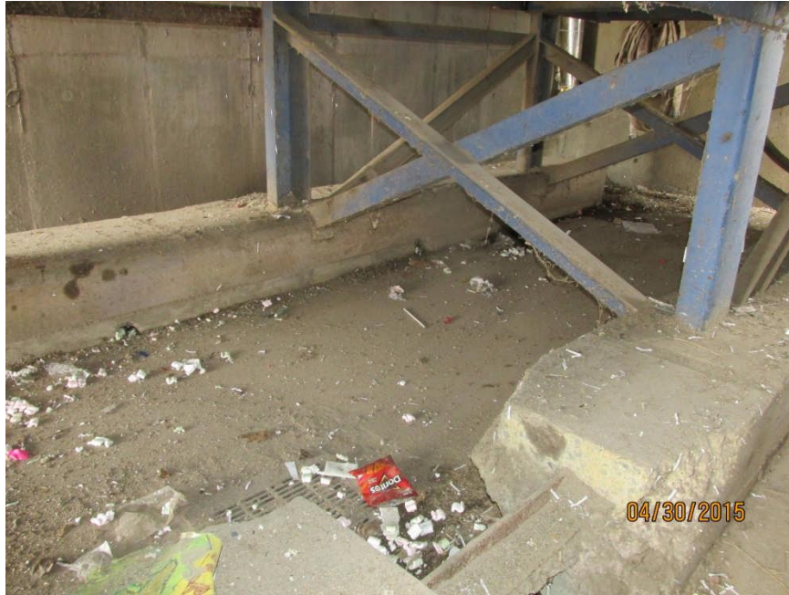
Photo #9 – Lower Level Floor below Compactor: compactor support steel encased in concrete curbs.
