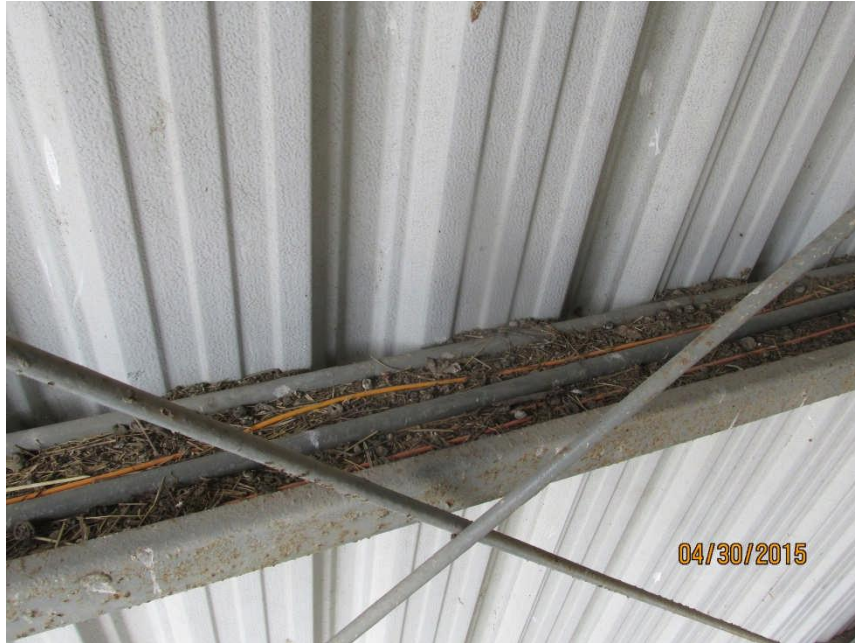
Photo #7 – Upper Level North Wall: horizontal girt and X-bracing with corrosion, peeling paint, and debris.
